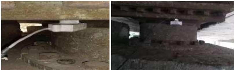
Picture 12. Sensor Under The Bridge.
