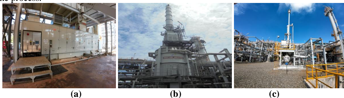
Figure 1. The Gas Turbin Generator (a). The Oil Heater (b). The DHU Reboiler (c).
