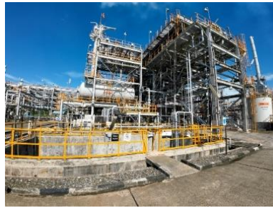
Figure 3. Acid Gas Removal Unit.
